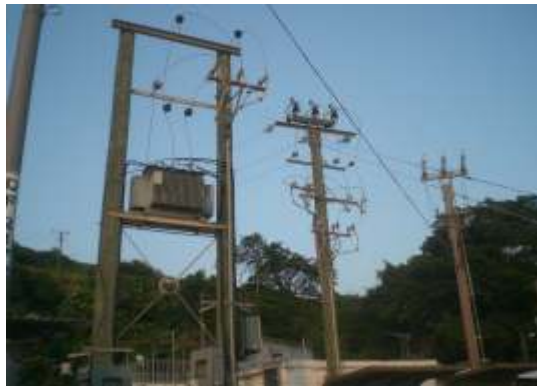
● Electricity pole transformer
